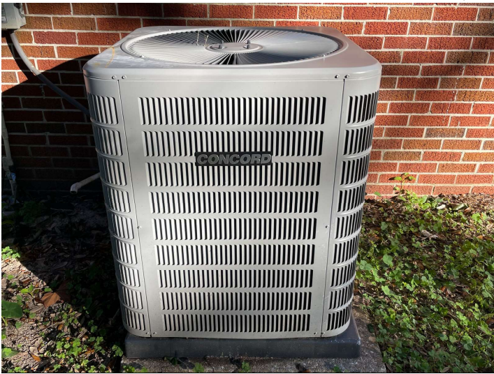
Condenser Unit (Located on left side of house)
