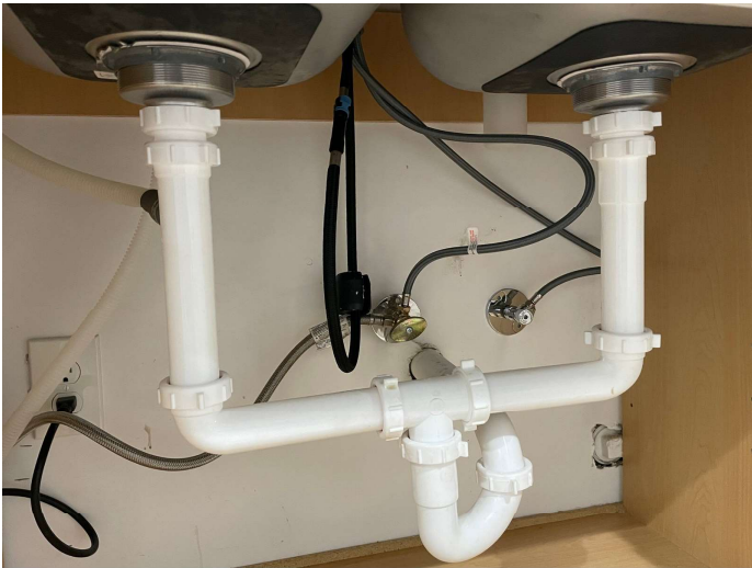
Kitchen Sink Supply valves and Drains
