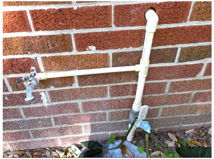
Main Shut Off Valve
