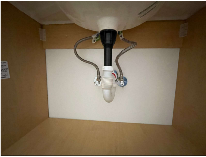
Bathroom 2 Sink Supply valves and Drains
