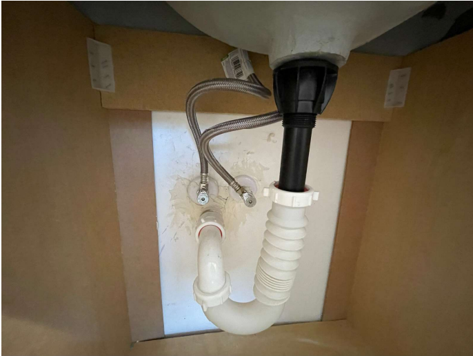
Bathroom 3 Sink Supply valves and Drains
