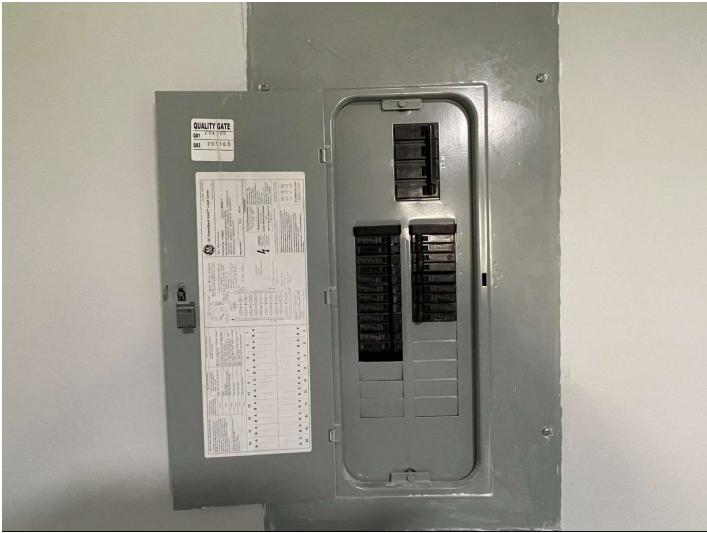
Sub-Panel (Located in Laundry Room)
