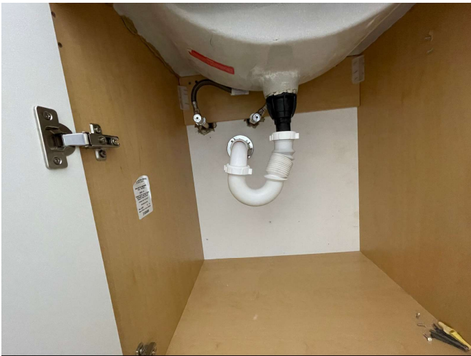
Bathroom 1 Sink Supply valves and Drains
