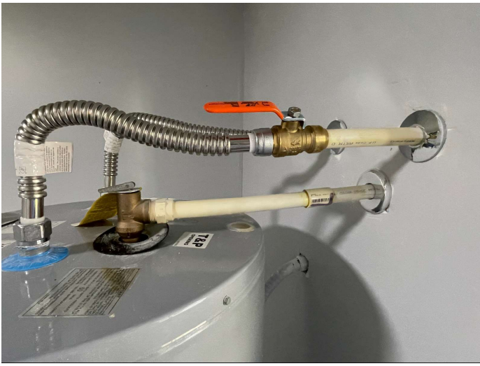
TPR Valve Drain Line (Supply lines CPVC)
