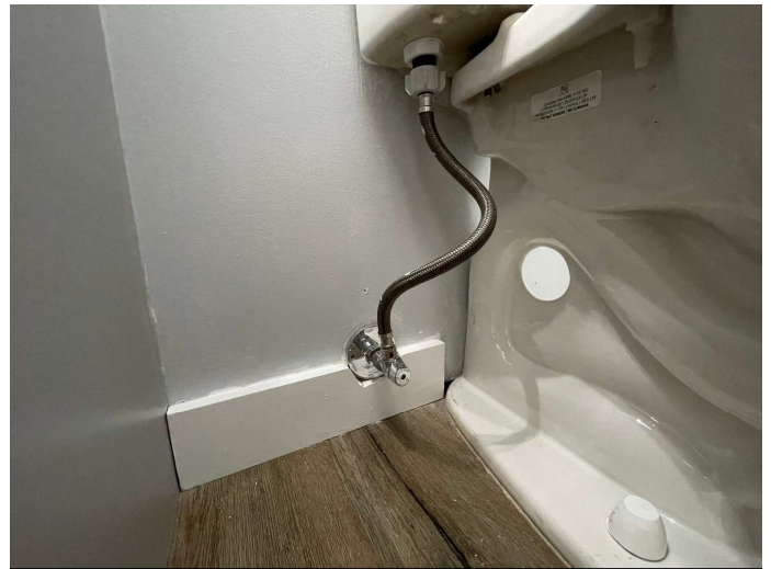
Bathroom 1 Toilet Supply valve
