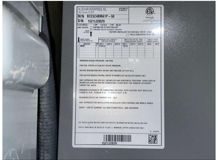
Air Handler (Manufactured November 2021)
