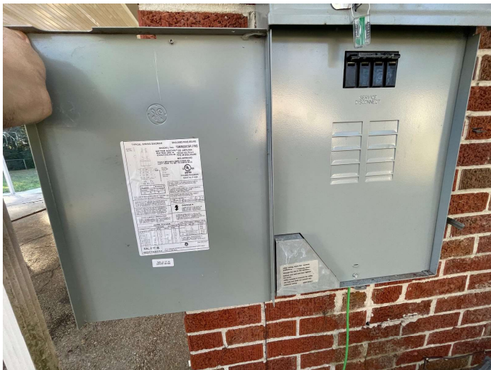
Main Panel (Located on Right Side of House)
