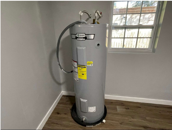
Water Heater (Located in Laundry Room)
