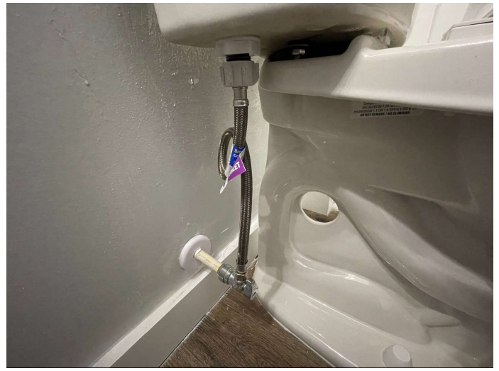
Bathroom 2 Toilet Supply valve
