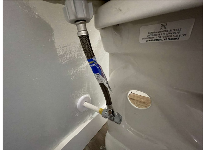
Bathroom 3 Toilet Supply valve
