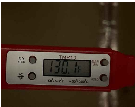
Supply Air Temperature
