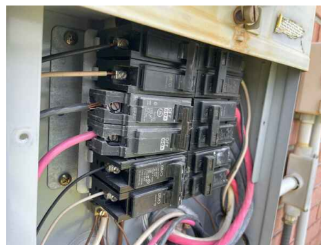
Left Breaker View
