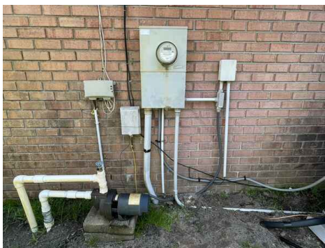
Main Entrance Panel
