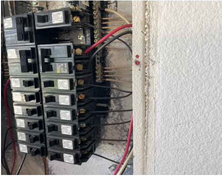
Right Breaker View
