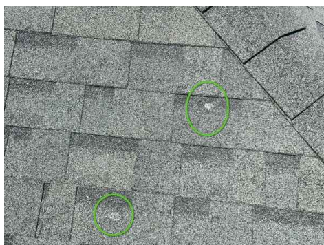
Appears to be Hail Damage (Multiple places over roof)
