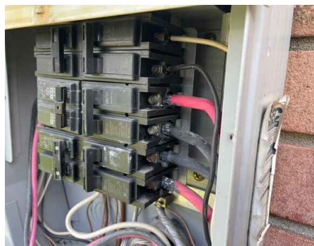
Right Breaker View
