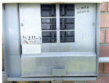
Main Disconnect (All six breakers must be off to stop flow of power to house) Any new homeowner should familiarize themselves with this process.
