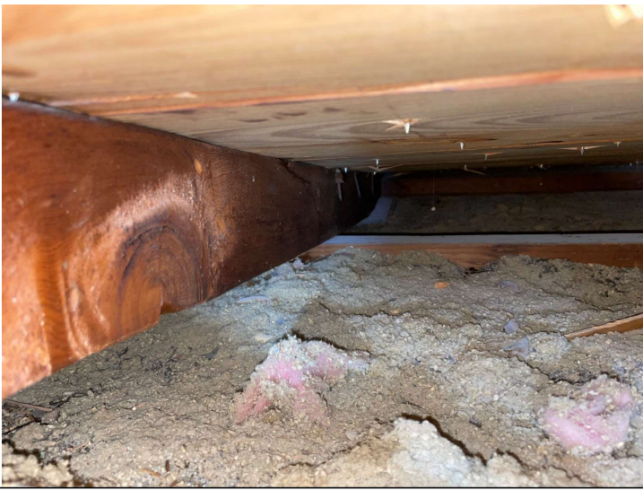
Roof To Wall Connection (Appears to be toenails only)
