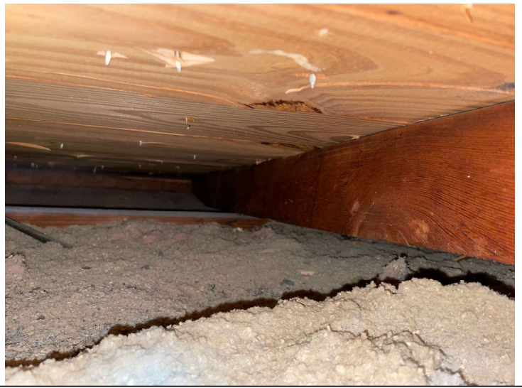
Roof To Wall Connection (Appears to be toenails only)
